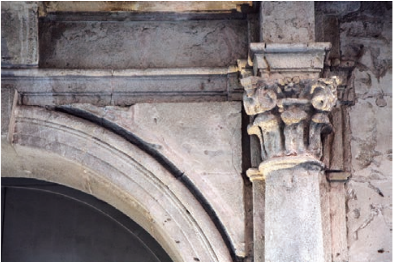
Fig. 2. Detalle arquitectónico de la puerta principal / Architectural detail of the main door, MUBAG, 2023
